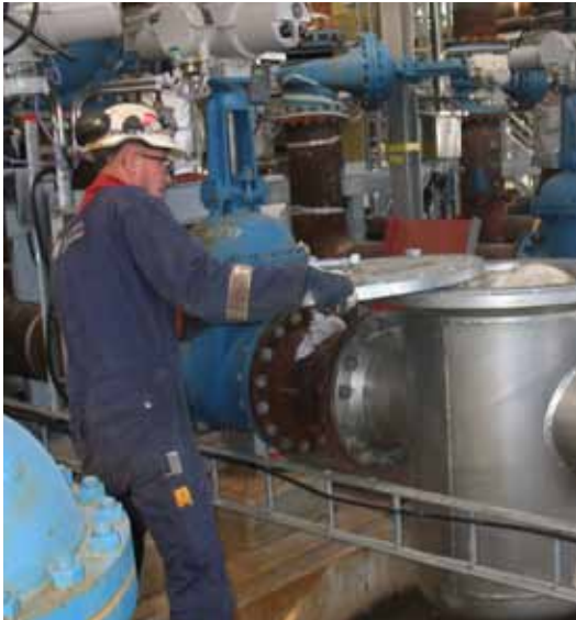
Filter change at a pump house
