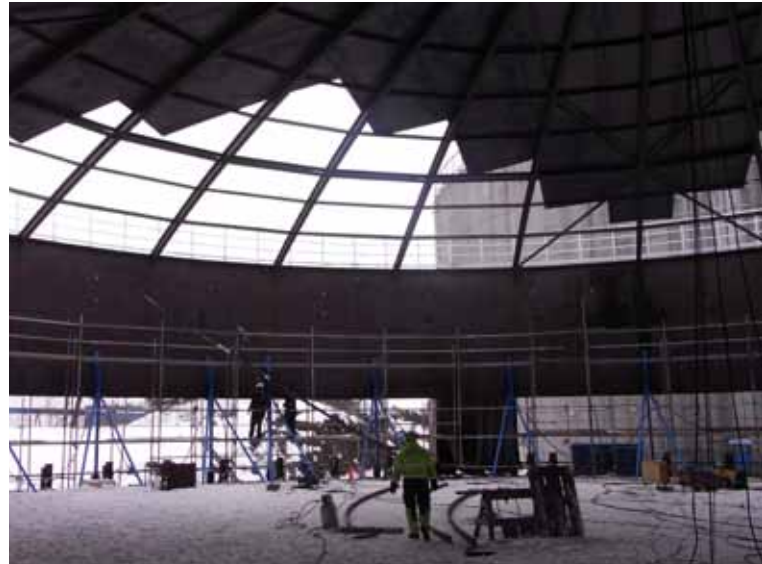
Inside Vopak's Tank in Gothenburg
